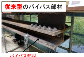
Fig.1 Corrosion of joint
