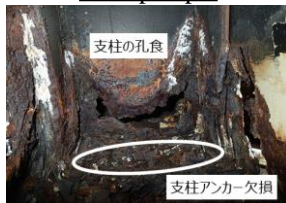
Damage of steel parapet
